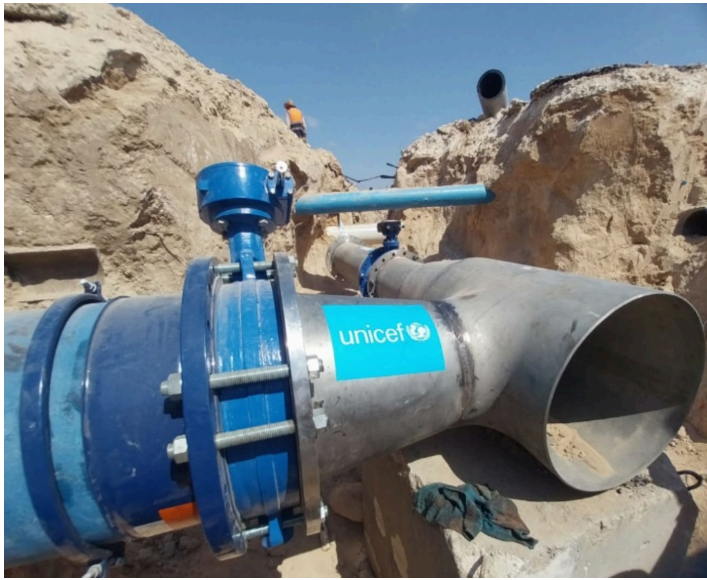
UNICEF restored the Bani Said water pipeline – providing 15 million litres of clean water per day to 300,000 people in Deir al Balah, Al Zuwayda and Al Bureij in the central Gaza Strip.
